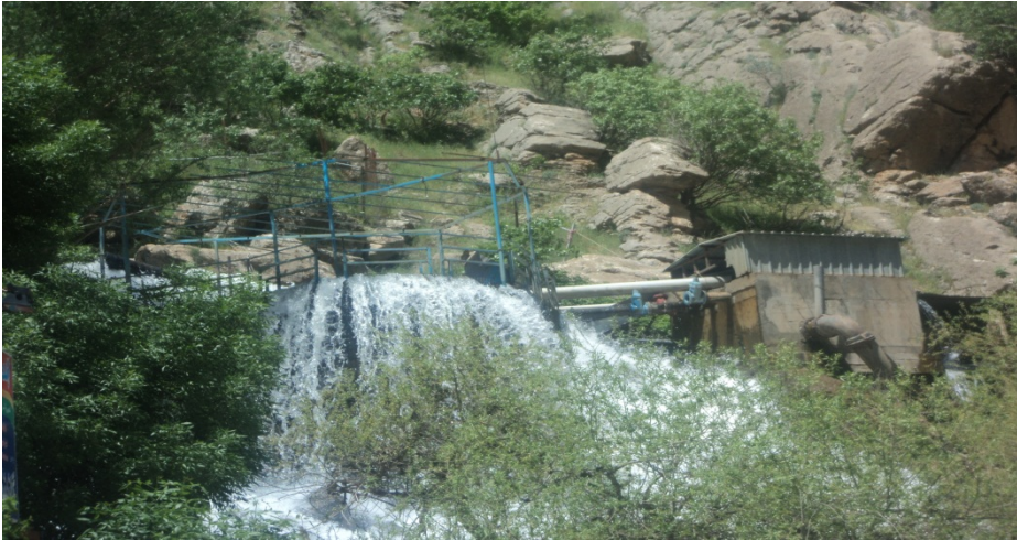
Figure 17. Shows the intake and the penstock (pipeline) of Bekal water treatment plant
