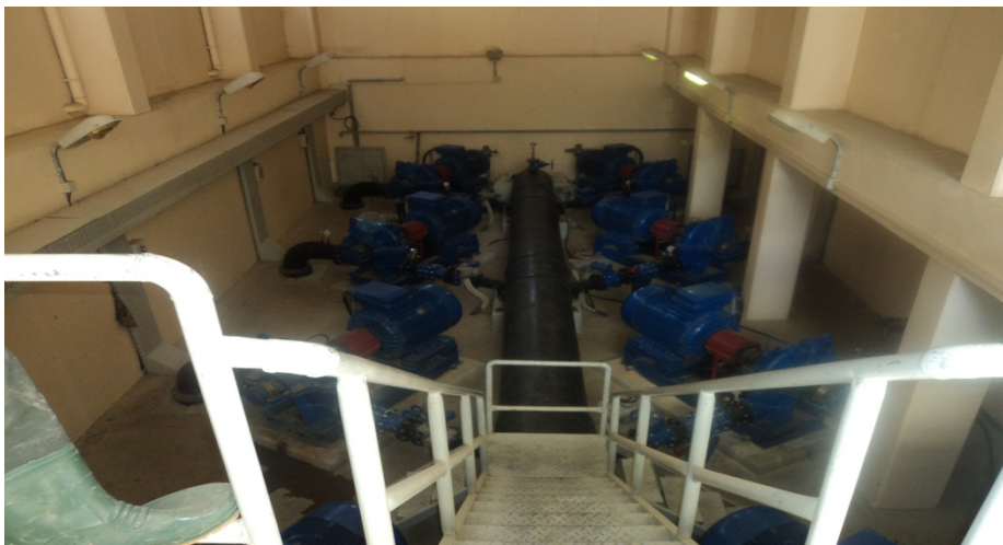
Figure 18. Shows the high head pump station
